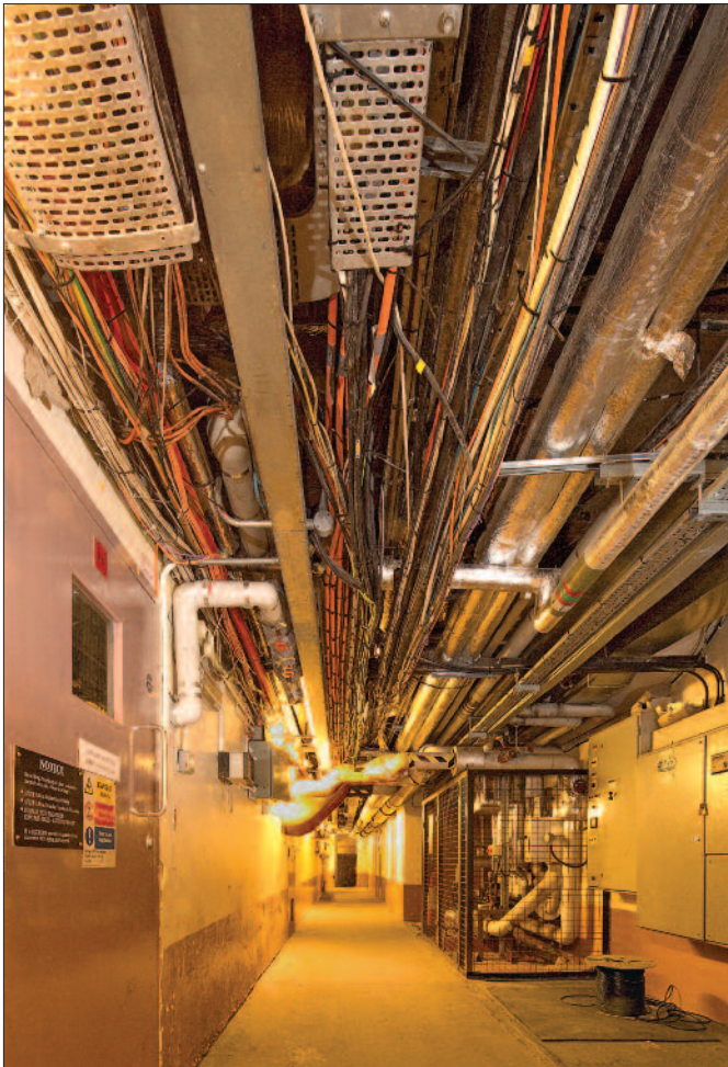
Ageing steam and electrical systems side by side are unsafe and often fail (Images © Parliamentary copyright)
