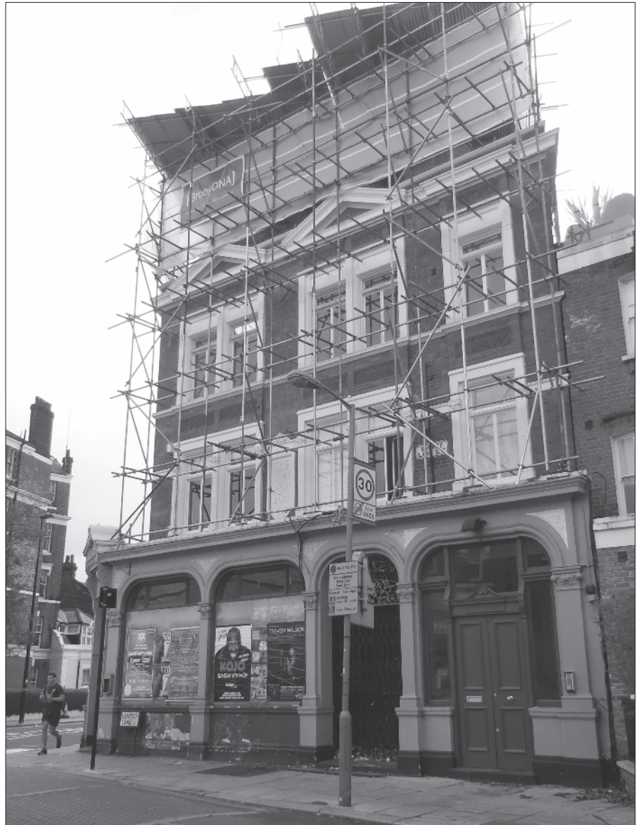
The Prince of Wales Battersea Bridge Road awaits conversion to residential flats plus a 4-bed detached house in the former garden
