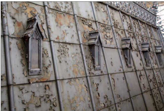
A cast iron roof covered in rust and peeling paint (Images © Parliamentary copyright)
