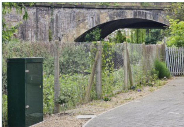
The north side of 'tunnel' with the brick archway; the proposed cantilevered walkway would be to the right hand side above the river
